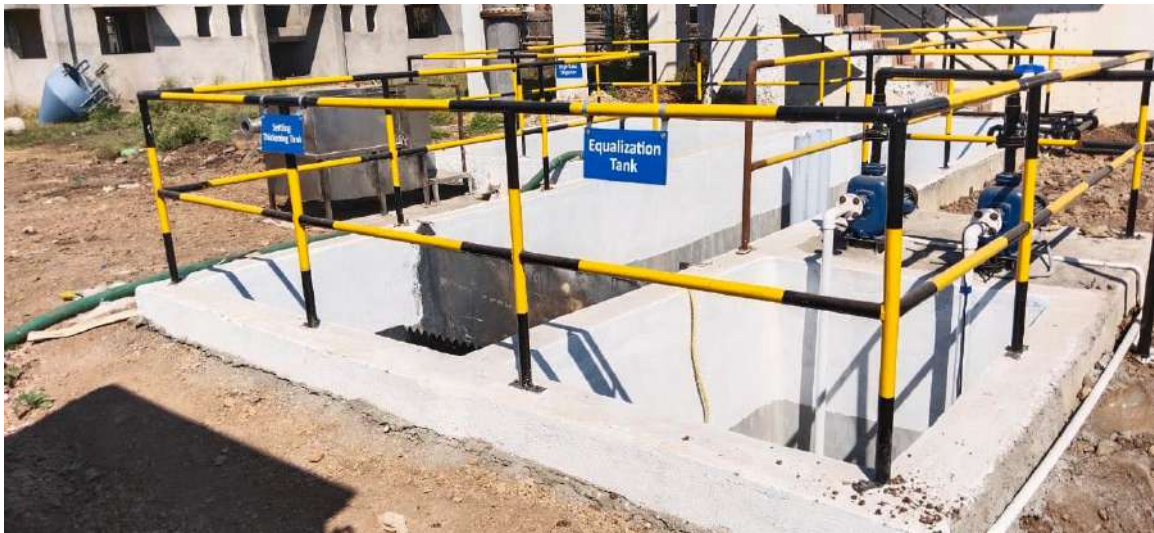
Figure 27: Newly added Secondary Co-Treatment units
