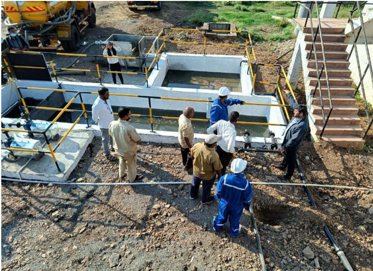
Figure 25: Training by ESF to STP operators
