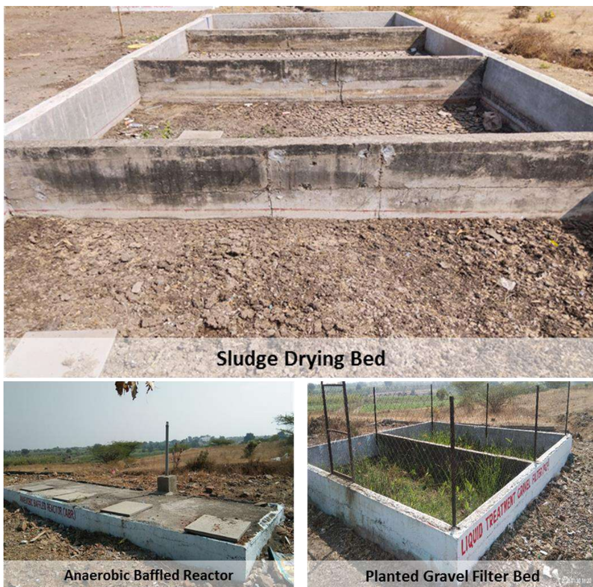
Figure 17: Treatment Units at the FSTP in Indapur
