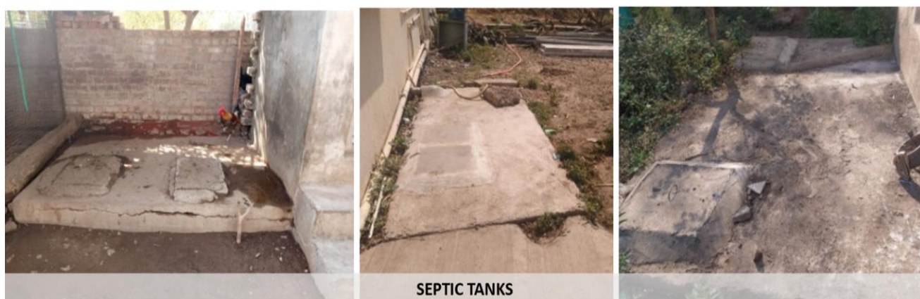
Figure 15 Septic Tank (Rural)
