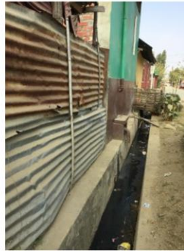
Lined, open drains
