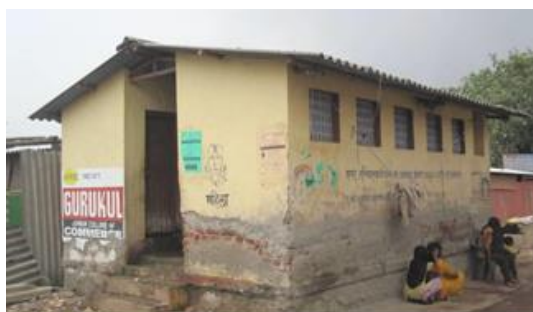
Figure 3: Rapid Deterioration in New Block
